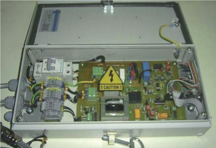
Control panel interior
